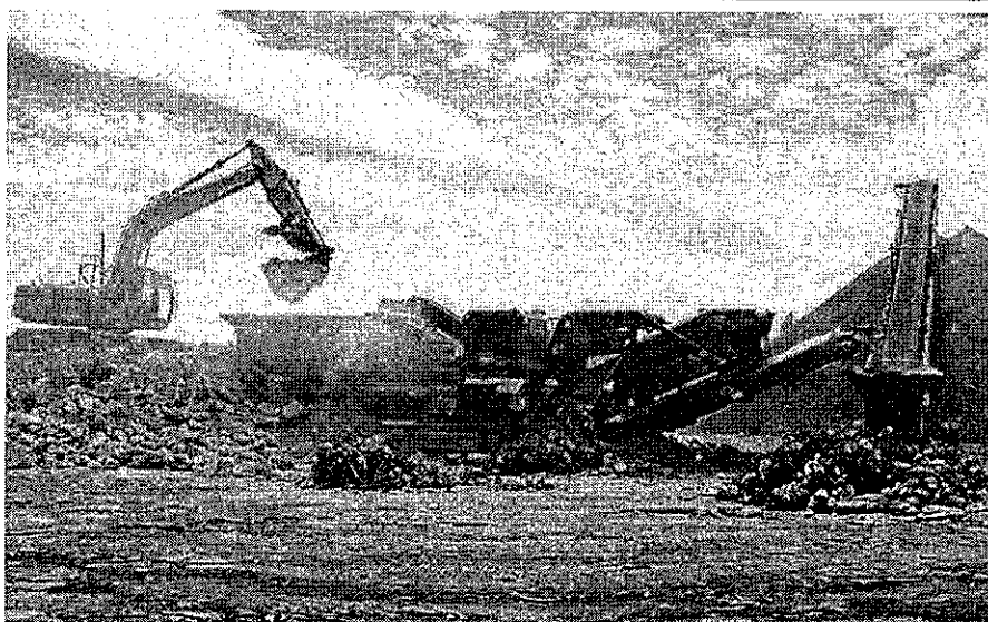
An excavator dumps cement pieces into a grinder at Peña's Material Recovery Facility in Cutler Monday afternoon. The company has increased the county's construction and demolition material recycling rate. / Luis Hernandez
